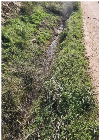
Figure 7.3.4.6. Appearance of the lateral slope of the third pond; the run-off of the liquid waste produced by the overflow and seepage of the third pond can be seen.
